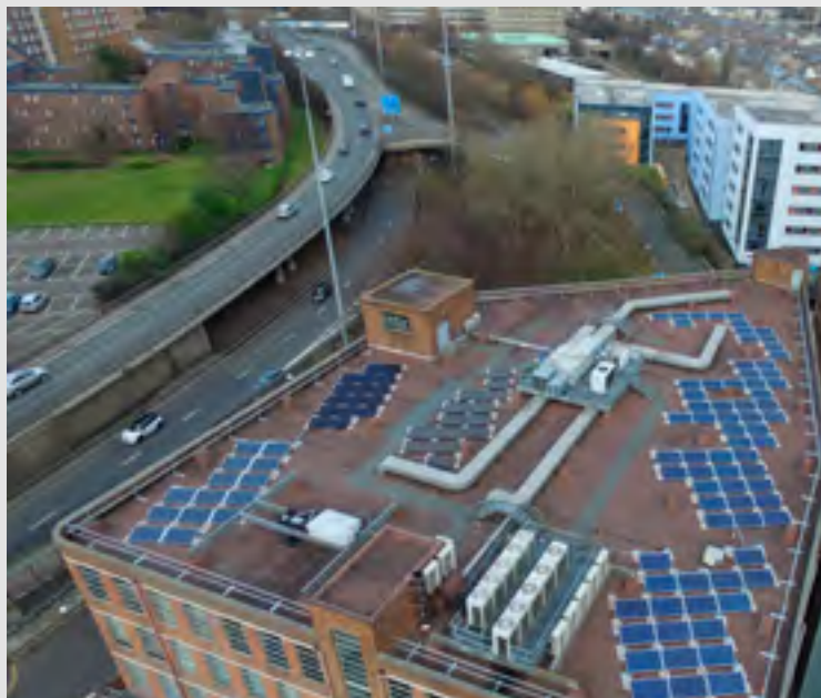
The solar panels on the roof of Pandon Building.
